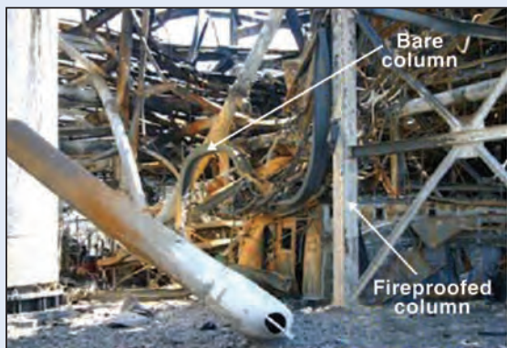
FIGURE 5. Collapse of non-fire-protected structural steel
